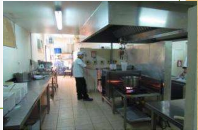
Kitchen unit for CECC at Al Ruwais
